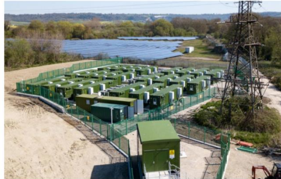
Zenobe grid battery storage site in Aylesford, UK. The company recently also got involved in the transport sector with an electric bus deal (below). Images: Zenobe.
