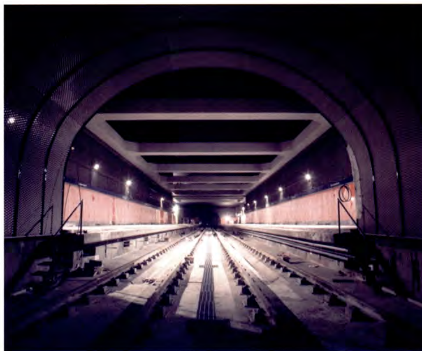
Internal view of El Casar station.
