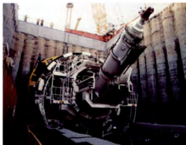
View of the screw conveyor
